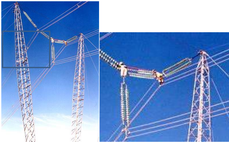
Figure 6-80 Electrical test of simulated maintenance on a compact 400kV inter-phase assembly 8
