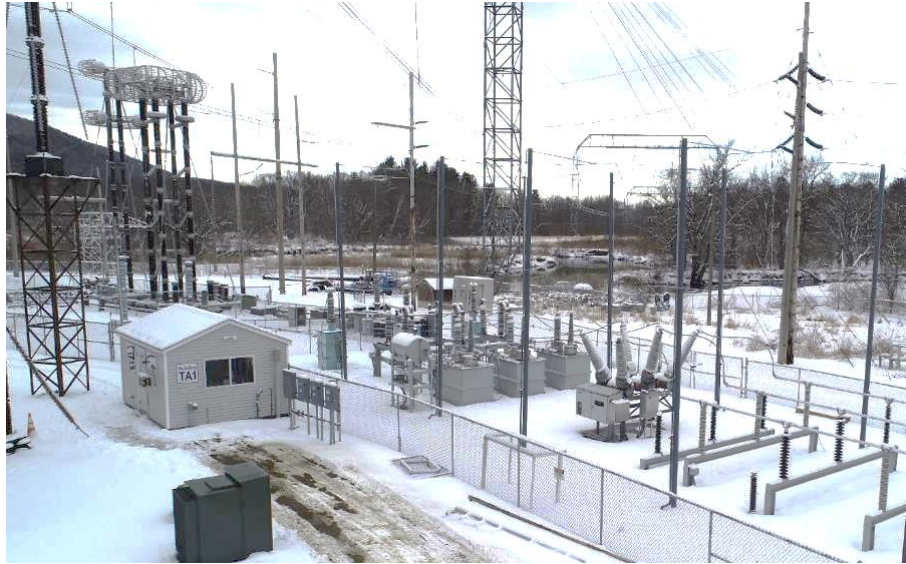
Figure 6-43 EPRI's full-scale 138kV research substation for industry testing of transformer monitors
