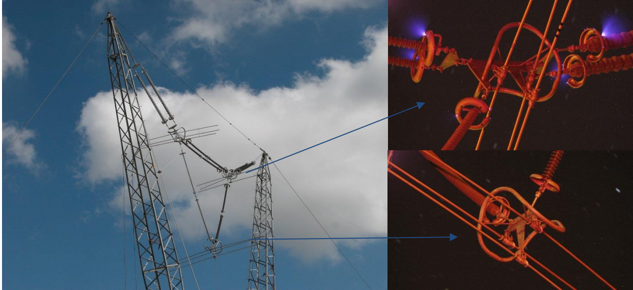
Figure 6-79 Electrical test arrangement for compact 400kV assembly 8,13
