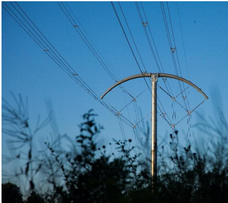
Figure 6-73 BOLD tower (Courtesy of BOLD Transmission, LLC)
