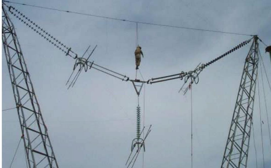
Figure 6-81 Electrical test of simulated Live Maintenance of 400kV crossrope tower [15]
