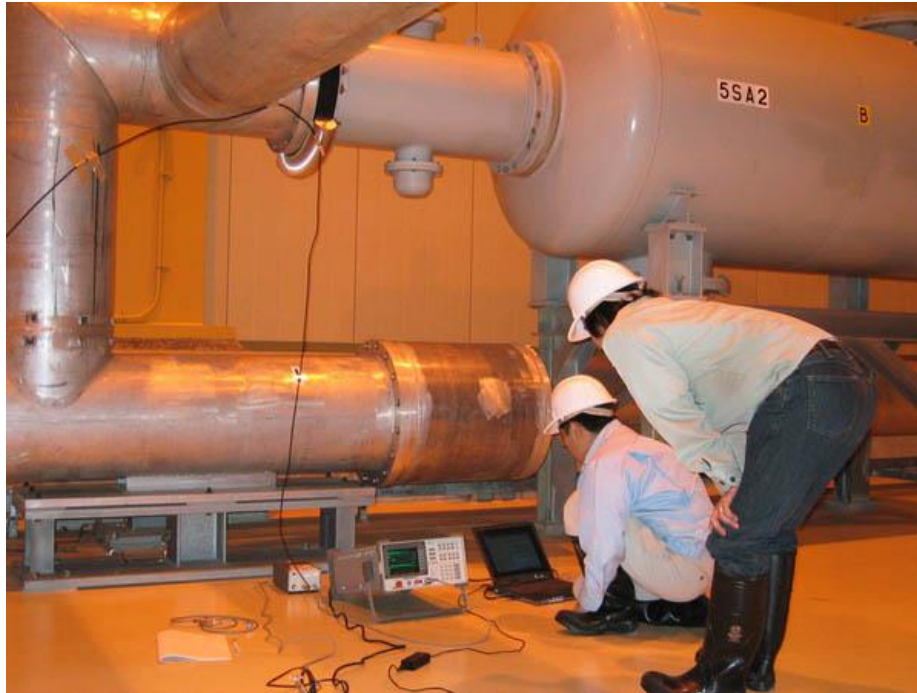
Figure 6-90 UHF being applied in the field. In this case, coupling was via a barrier since there were only a few window ports.
