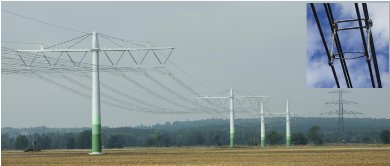
Figure 6-61 Vertical compaction of double circuit line [Courtesy of 50hertz Transmission/ SPIE SAG]
