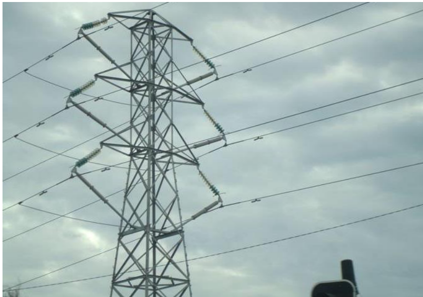
Figure 6-68 66 to 110 kV line upgrade
