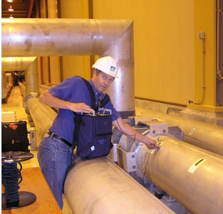
Figure 6-91 Acoustic Emission (AE) being applied to a section of GIS bus.
