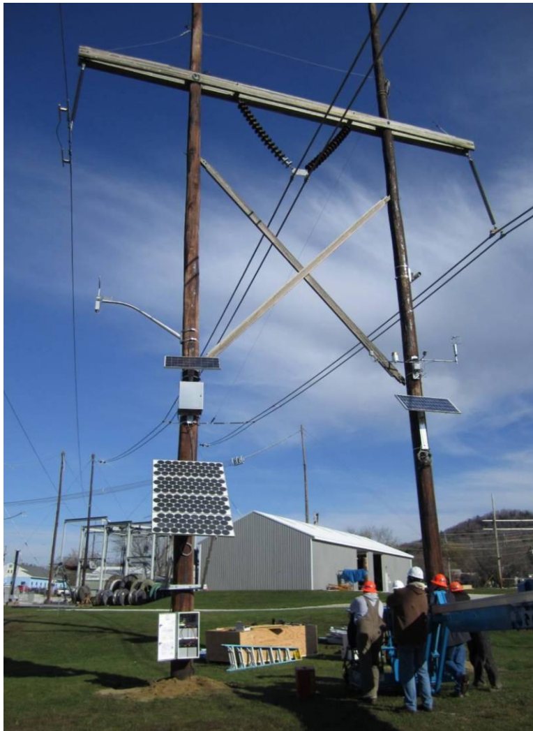
Figure 6-10 Utility line crew practicing installation of line ratings technologies at EPRI High Voltage Laboratory
