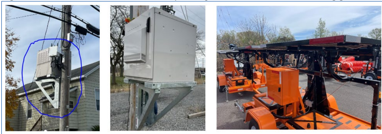
Figure 2.12.3 Pole Mounted extended battery backup solution and mobile connecting grid router
