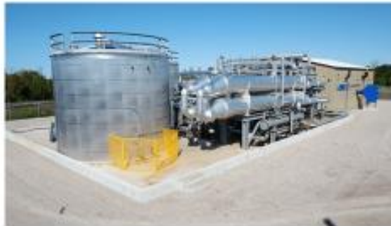
Compressed Air Energy Storage
