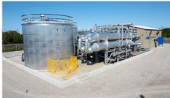
Compressed Air Energy Storage
